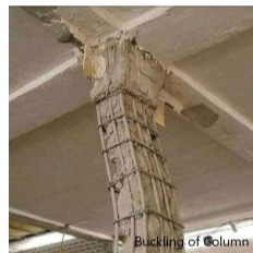
Buckling of column
